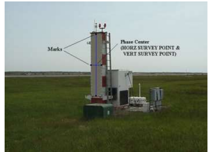
ILS ELEVATION GUIDANCE STATION
